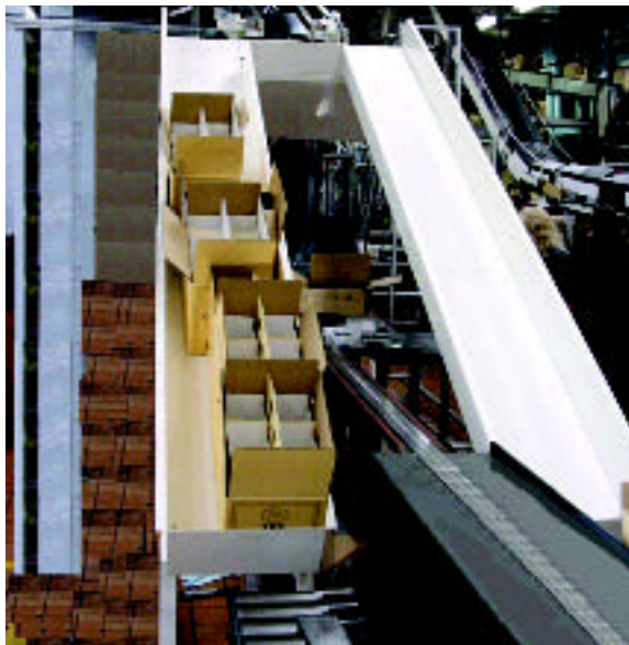
Conveyor Systems: Empty case feeding system for Chivas
