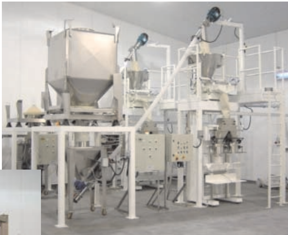
In-IBC blending: Matcon mixer (left) and filling system (above) at Sleaford Quality Foods
