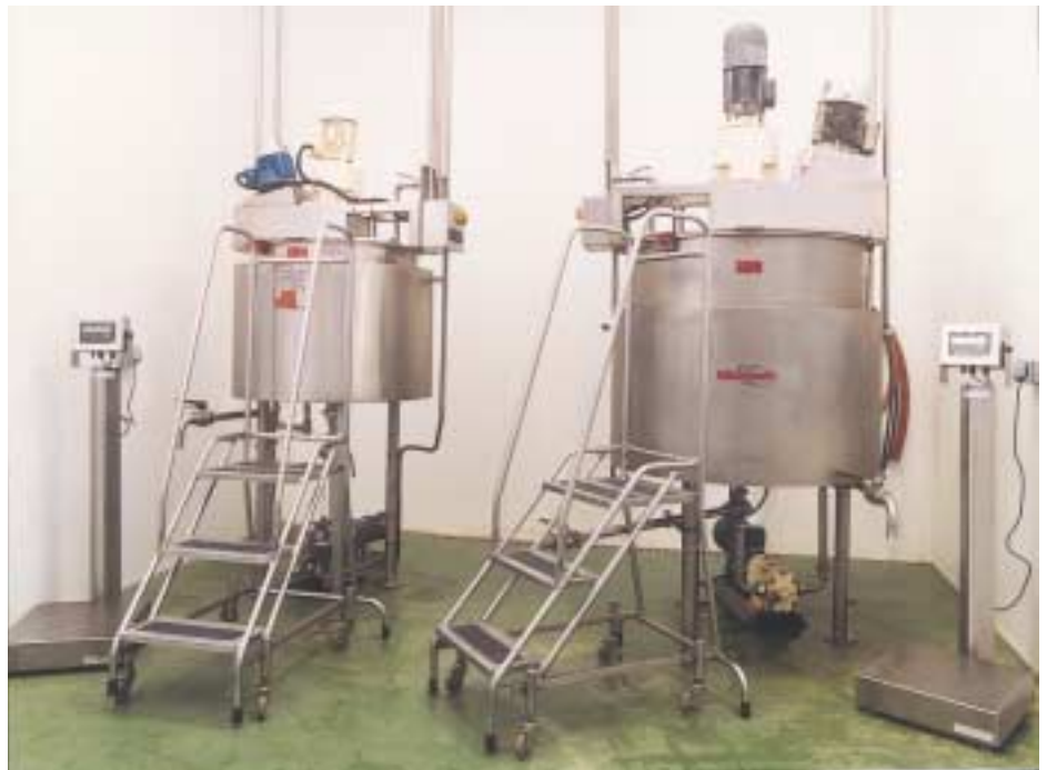
Liquid mixing: Welcome uses a range of vessels from 250 to 500 litres, with a variety of mixers for versatility
